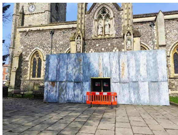
The Ugly: corrugated iron shrouds the South porch
