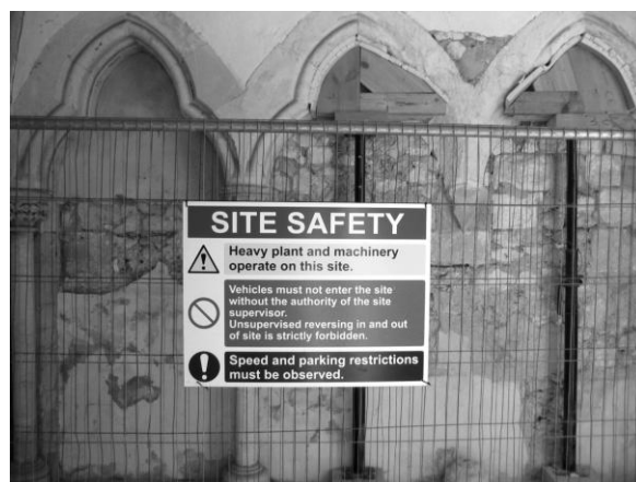
Sign of the times. The perceived need to restrict vehicles driving at speed inside the porch may cause a smile, but the clear damage to the fabric of building behind is worrying.
