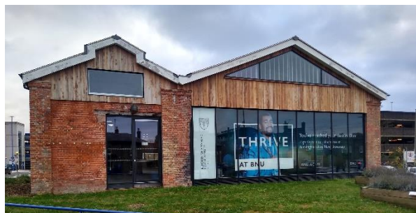
Already paint is peeling from the top of the façade. Will it ever come to life as planned?
